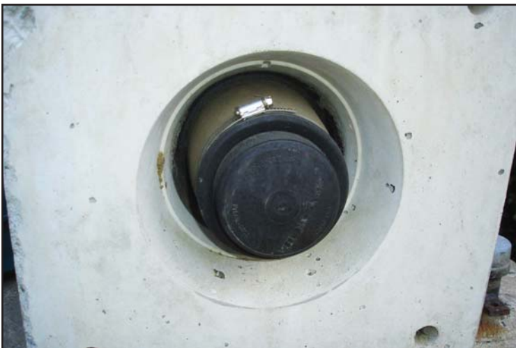
Polylok Boot Seal properly installed.
