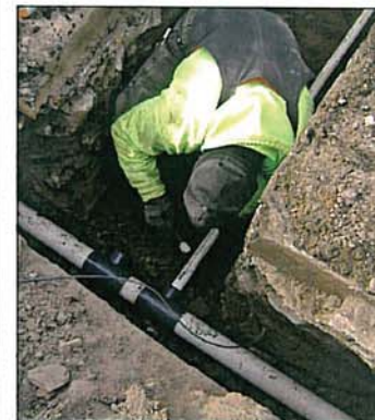
A worker from Dan Cristiani Excavating connects a service lateral to the force main.
